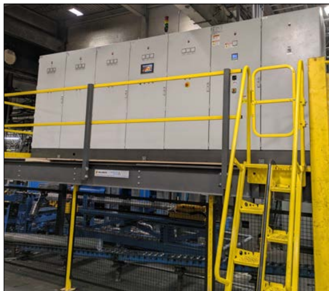
Figure 2. The IGBT converter allows for better temperature control in the furnace.
