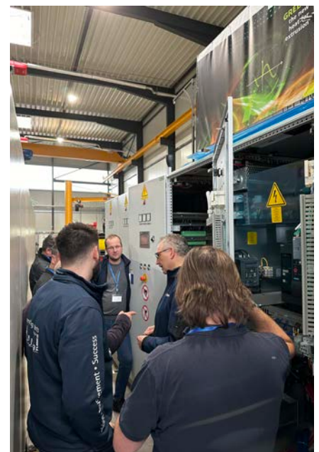
Figure 4: Showing of the new power electronics during the customer event (Source: extrutec)
